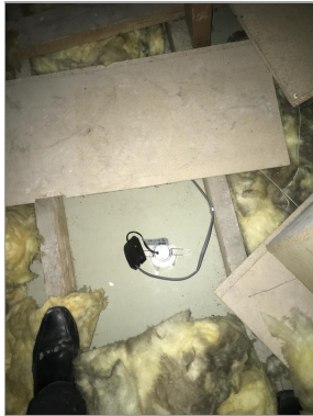
Photo - 8 No insulation over lighting
