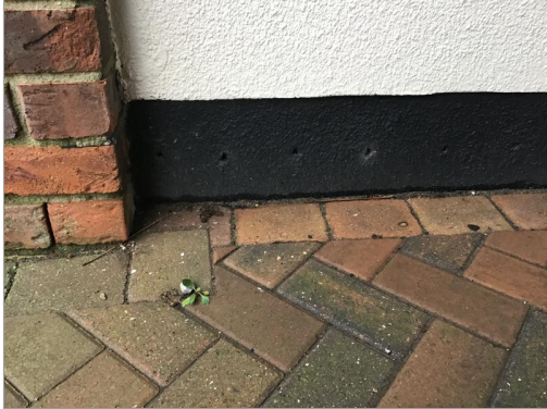
Photo - 3 Evidence chemical DPC
