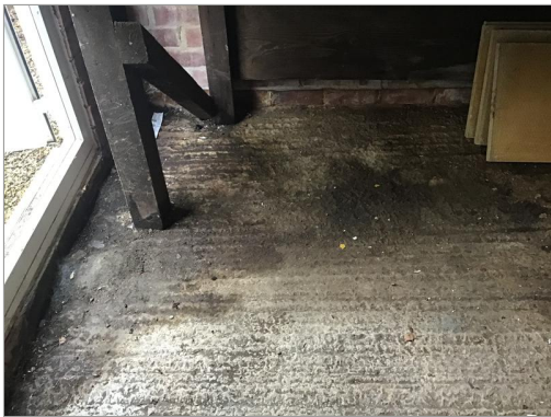
Photo - 15 Damp in garage floor
