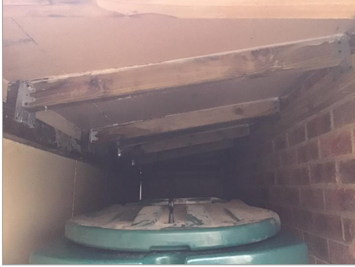
Photo - 13 Oil tank
